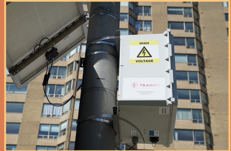
Train detection sensor installed at the Richmond St rail crossing
